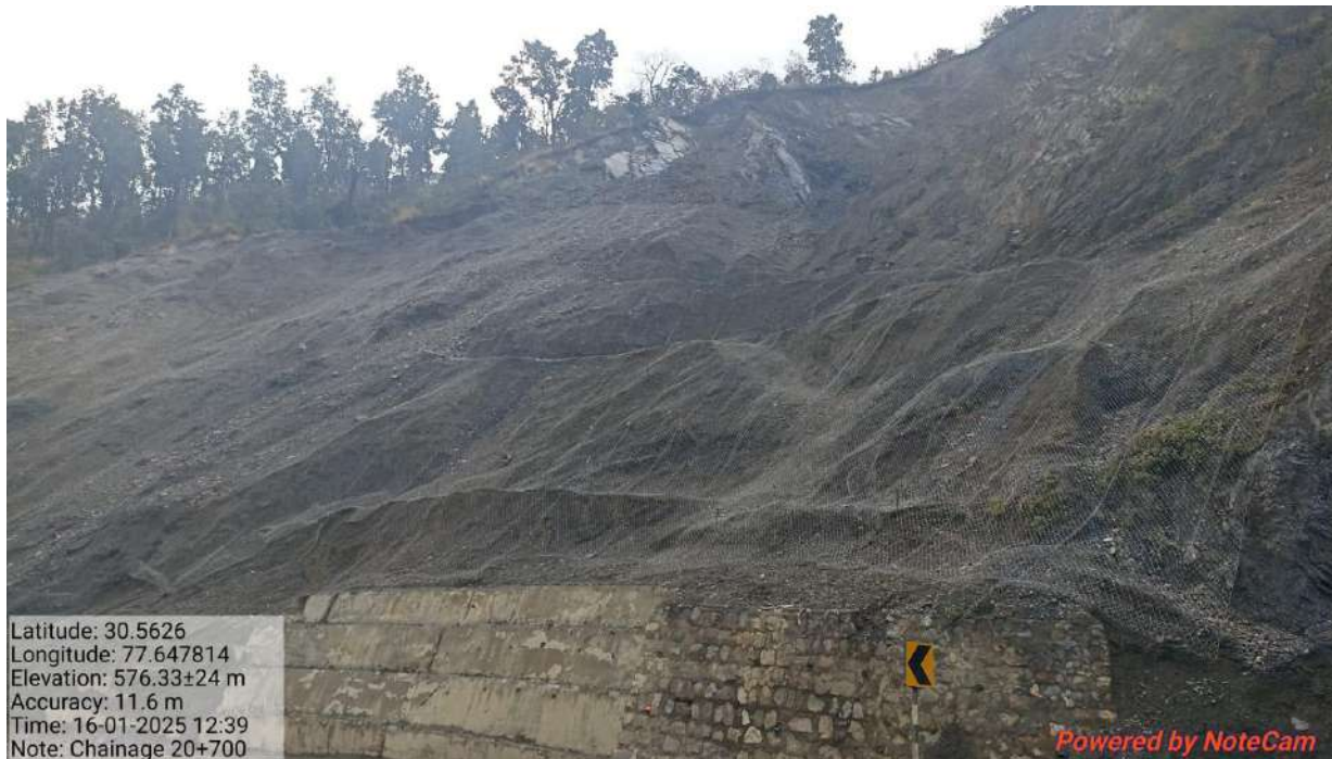
Refer photo at Page No. 4391 (Second Photo): During the rainy season, landslide at the hillside had occurred with big size of boulders. No dumping has been done.
